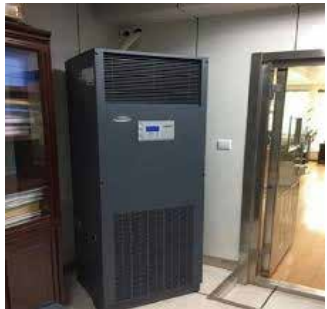
Precision Air Conditioning Unit Project Zong.
